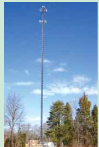
Figure 1 – A typical macrocell base station with receive antennae at the top, transmit antennae below the receive antennae, and the control system at the base.
